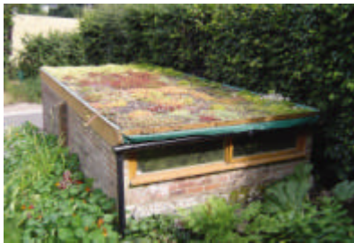
After stripping the roof, we laid a membrane over the existing chipboard, added sifted top soil & planted drought resistant sedum.
